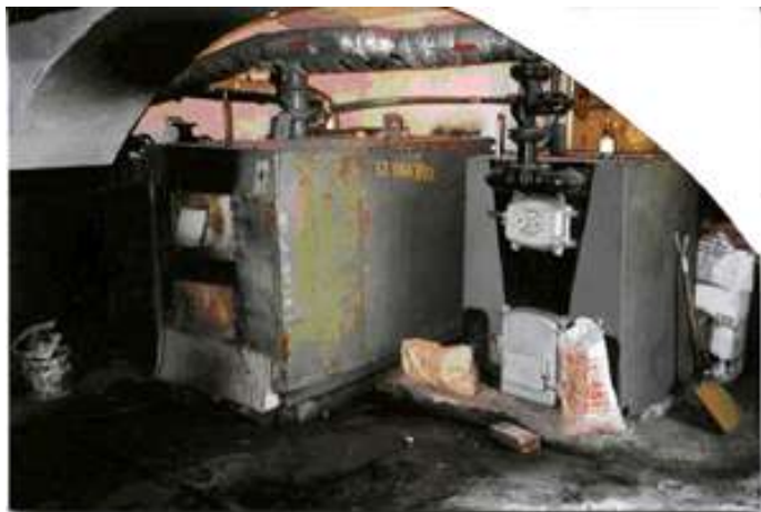
THE BOILER AT OKREZNA STREET BEFORE MODERNISATION
